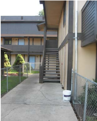
Side of Building 2 Stairs Not Code Compliant
